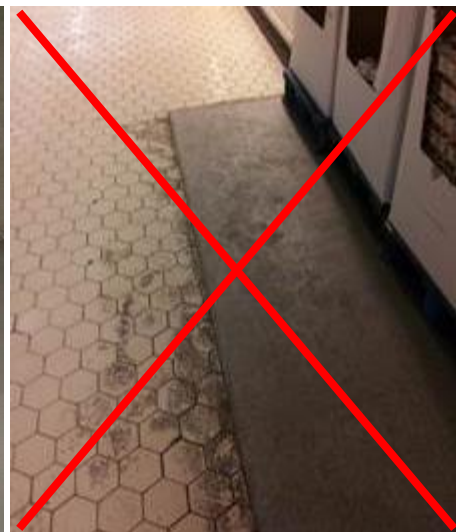
uneven, not suitable substrate
